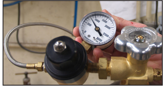
Fig. 33 Source tank pressure gauge
