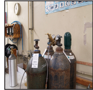
Fig. 35 Large compressed gas supply bottle
